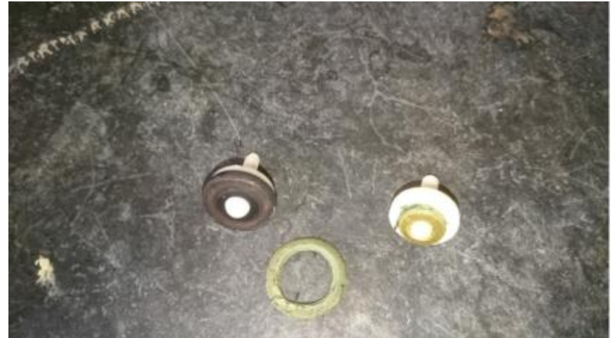
Washer on right from bath at house 16 - serious leak for considerable time- reseated and replaced by AEHW trainee
