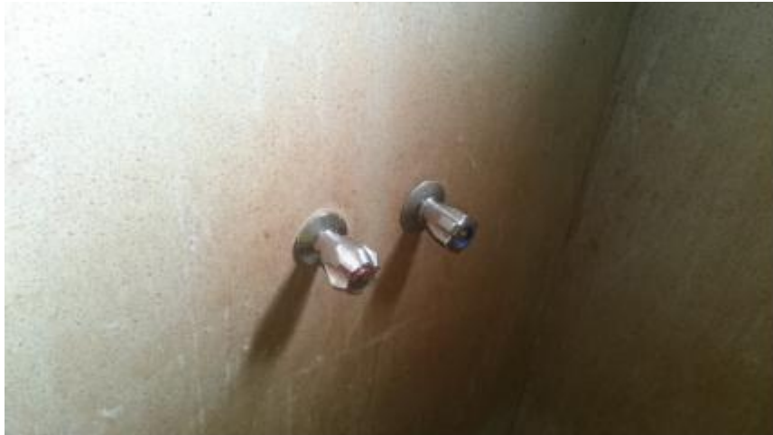
House 16 - shower tap spindle replaced ( previously no handle)
