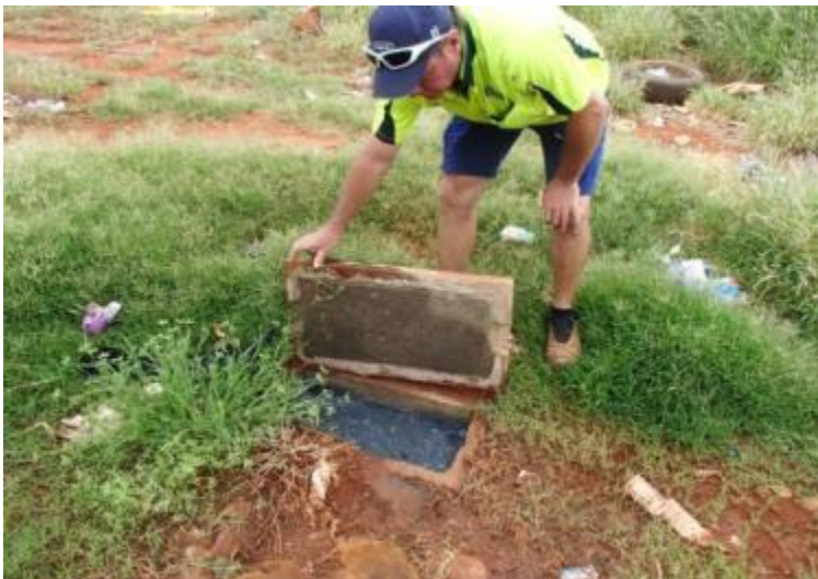
Complete System Failure
