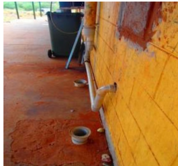
Very Poor 'Code' Compliance
